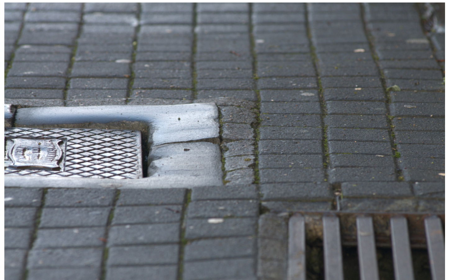
Fig. 5 Footpath showing the wear and corrosion that time brings. Mallow Street, Limerick, Authors own, 2013
